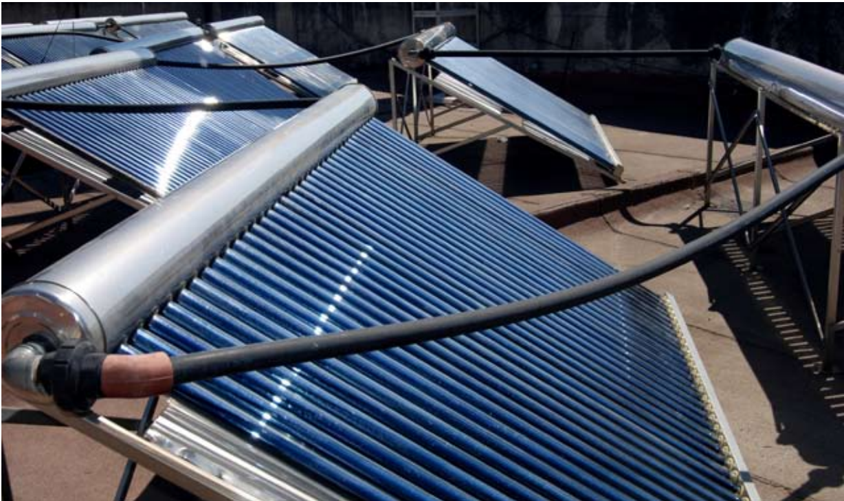
Illustration 7. Solar water heaters
