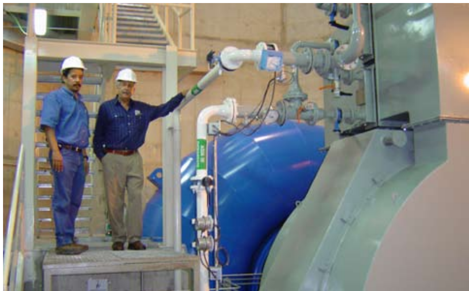
Illustration 8. Las Trojes small hydro project (8 MW)
